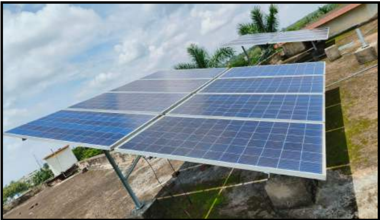
Solar panels on the rooftop of the Academic Building
