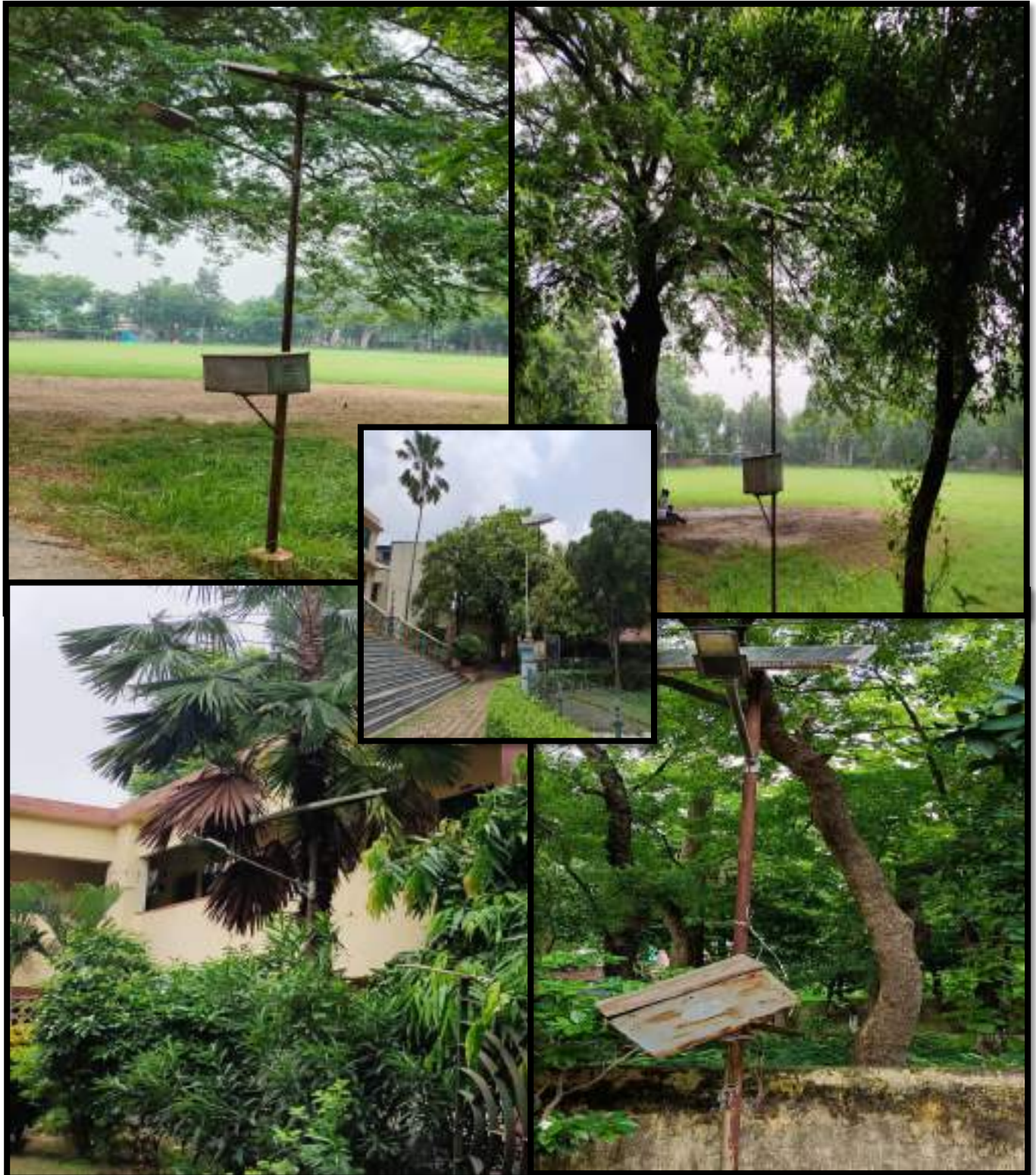
Solar Street Light at Hostel Campus
